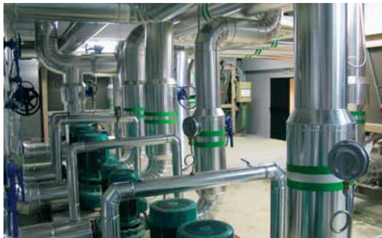
Central heating and cooling facilities at Teatro de El Escorial. Madrid
