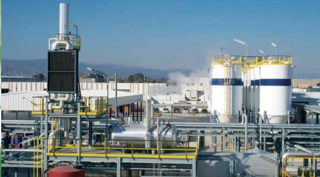
Full-service industrial waste treatment centre in Constantí. Tarragona
