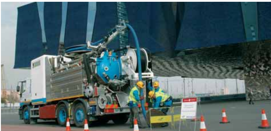
Vehicles combining vacuum pumps and water jets to clean sewer systems
